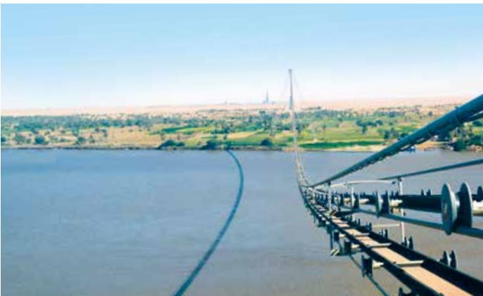
2011 A RopeCon® installation crosses the world's longest river, the Nile, which is roughly 850 m wide at this point.
