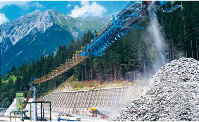
2001 The RopeCon® system is used for the first time. Between 2001 and 2004, the installation near Strengen, Tyrol, transports around 850,000 m 3 of tunnel excavation waste across an expressway, a railroad line and a river.
